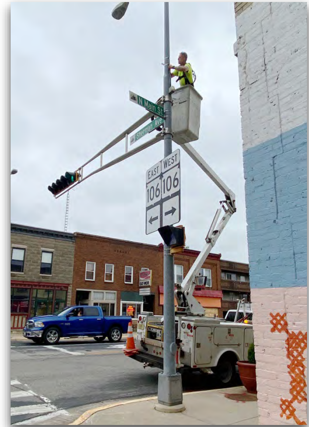
MEMBERS OF THE DEPARTMENT OF PUBLIC WORKS TAKE DOWN CHRISTMAS LIGHTS ON MAIN STREET.
